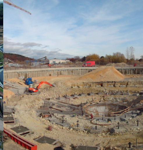
Steinhäule wastewater treatment plant, new sedimentation tank of the advanced treatment stage under construction
