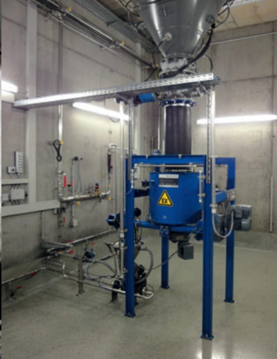
Kressbronn wastewater treatment plant, PAC dosing system
