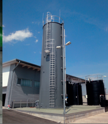
Lahr wastewater treatment plant, silo containing powdered activated carbon
