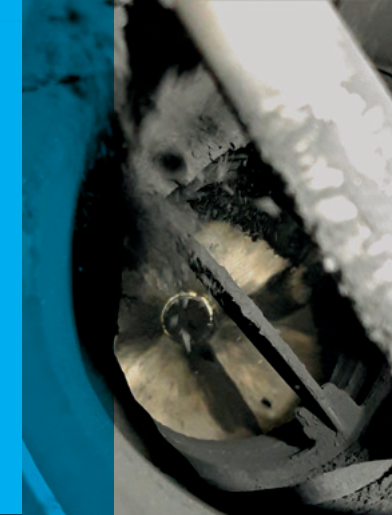
Wendlingen wastewater treatment plant, PAC dosing system
