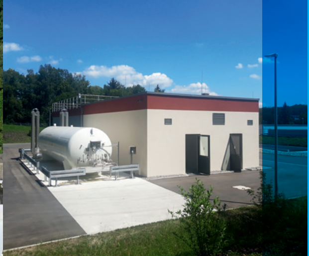
Eriskirch wastewater treatment plant that uses ozonation
