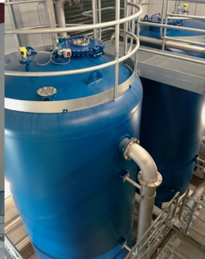
Westerheim wastewater treatment plant, GAC filter
