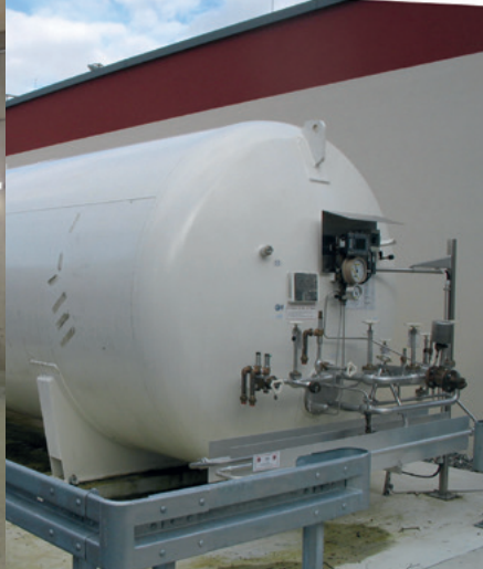
Eriskirch wastewater treatment plant, oxygen tank for the ozone system
