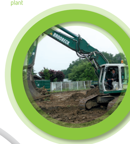
Ground being broken for the new filter building at the Westerheim wastewater treatment plant
